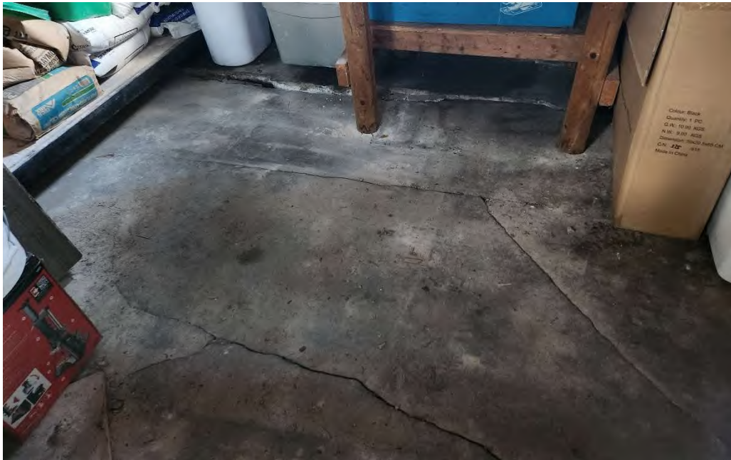
Cracked Concrete Slab
