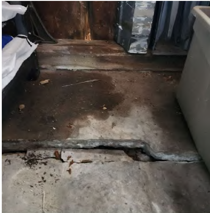
Deteriorated Concrete Slab and Untreated Bottom Sill Plate
