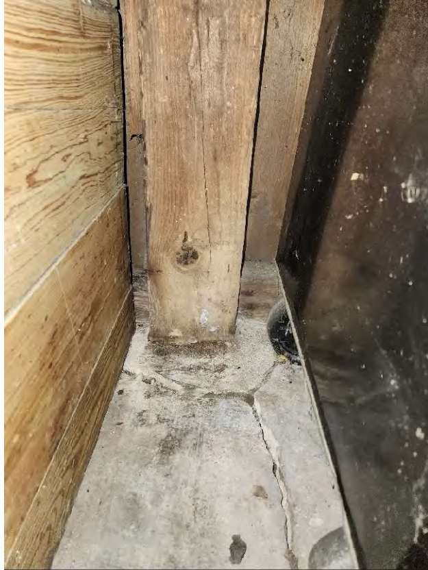
Main Wall Vertical Members (Untreated) Set In Concrete; Cracking Slab
