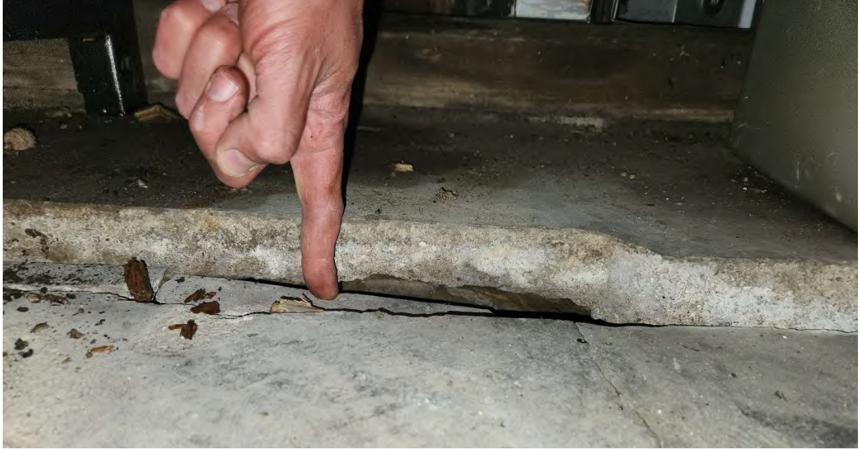
Deteriorated Concrete Slab and Untreated Bottom Sill Plate
