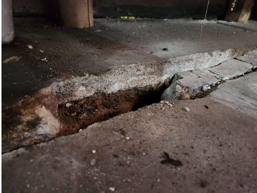
Deteriorated Concrete Slab (above)
