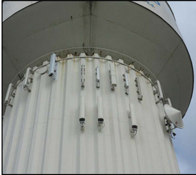
6 'Y' SECTOR ANTENNA MOUNT PHOTO SCALE: NONE
